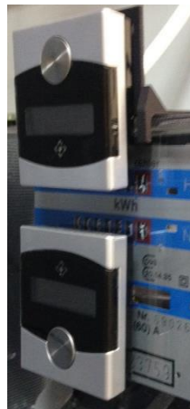
two EnergyCam devices on 2-Tariff Meter
