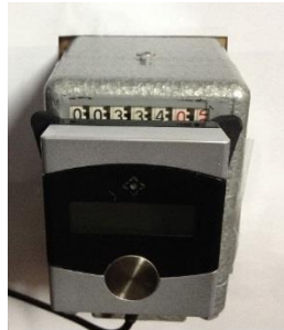
EnergyCam with mounted FAST Gas Meter Adapter on a Braun HZ5 oil meter
